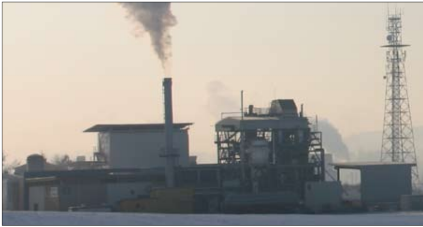
Figure 1 The Güssing gasification plant
